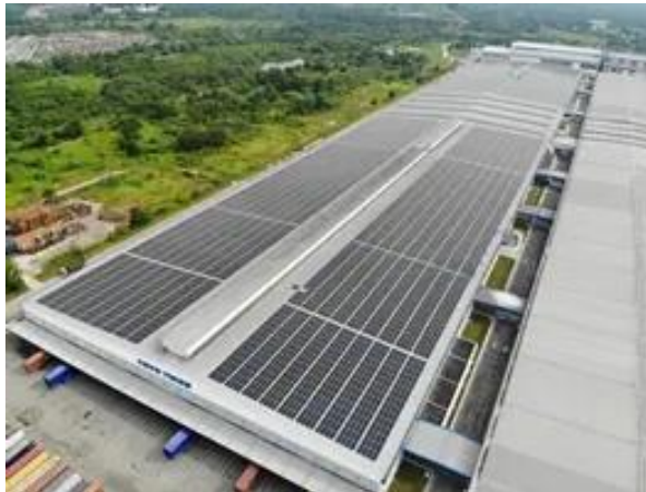
PV power generation system
