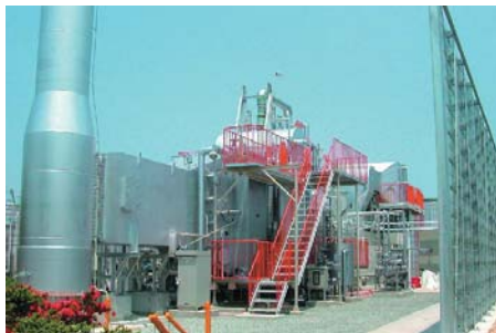
Co-generation systems that supply both heat and electricity are extremely effective in boosting resource efficiency at tire plants that use numerous heat sources. They are also an excellent means of reducing carbon dioxide emissions.
